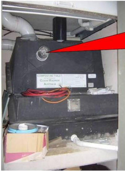
Newly installed container for excreta (Clivus Multrum)
