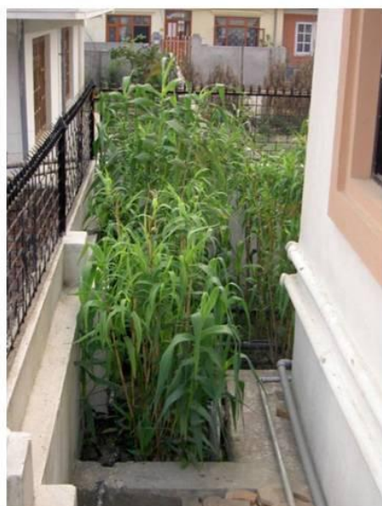
Reed bed for treating greywater that is recycled on the terrace
